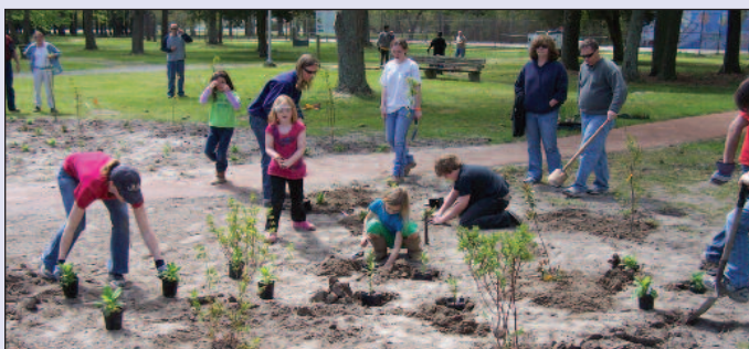
A rain garden is installed in Stephen Decatur Park, Berlin, to aid in stormwater runoff and flooding.
